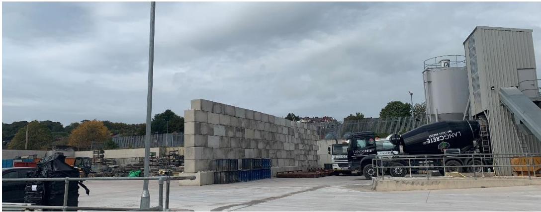
Figure Five – Photo showing acoustic barrier in place (taken 06/10/2022)
