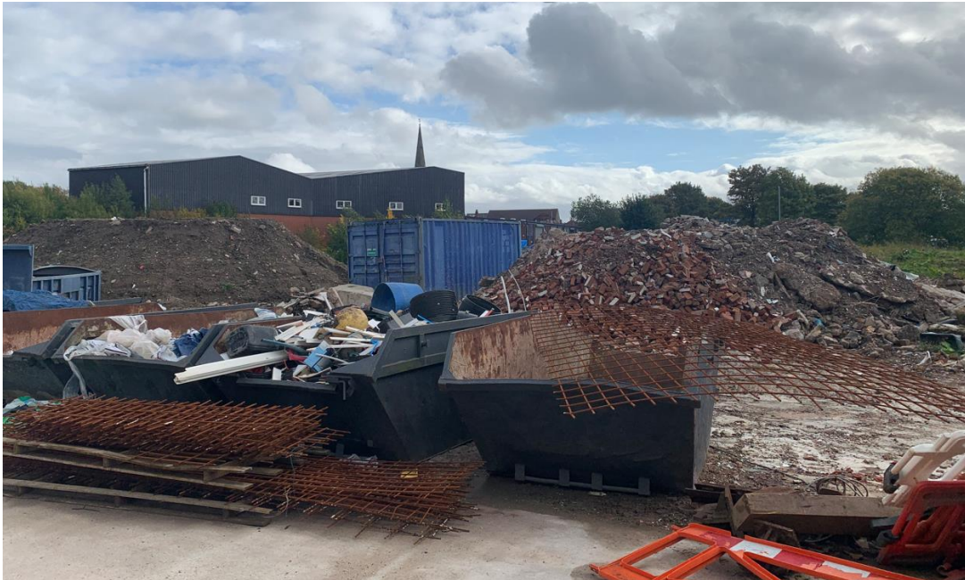
Figure Six – Photo showing construction waste deposited on site (taken 06/10/2022)
